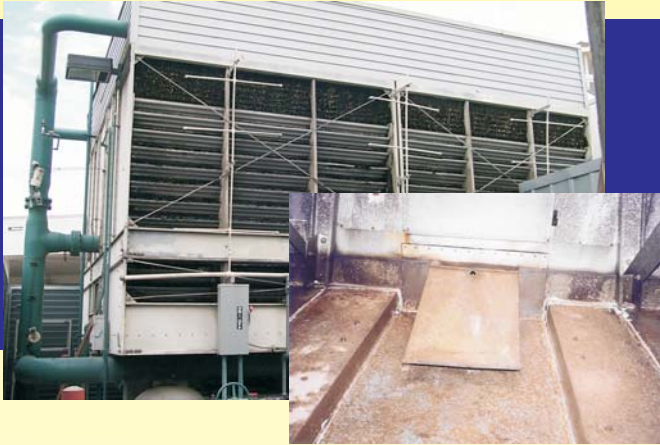
Tower basin in poor condition
